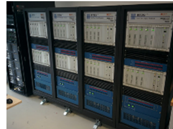
RTDS installation at the ACS Realtime Lab
