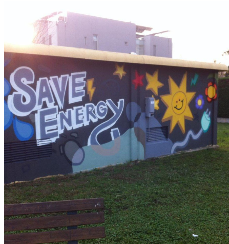
Unareti secondary substation in Brescia implementing the IDE4L substation automation unit
